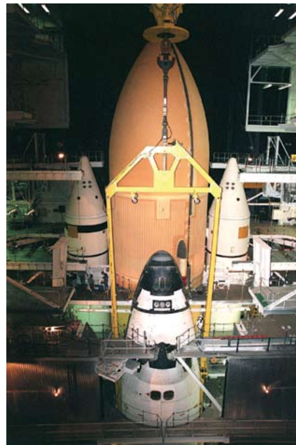
The elements of a space shuttle are integrated in one of the cavernous high bays of the Vehicle Assembly Building at Launch Complex 39. The platforms slide in and out, allowing workers to reach all levels of the vehicle. The orbiter is in the foreground. At the rear is the huge external tank, bracketed by solid rocket boosters.
