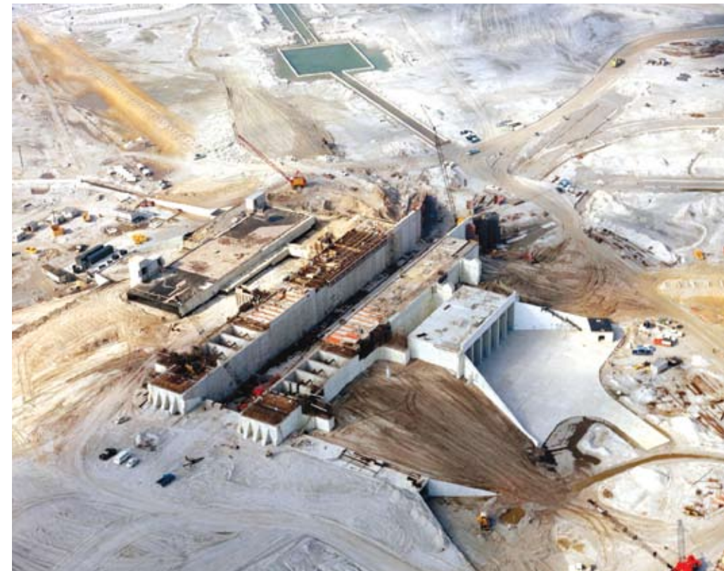
Construction of Pad A at Spaceport's Launch Complex 39. The pad hardstand contains 68,000 cubic yards of concrete.
