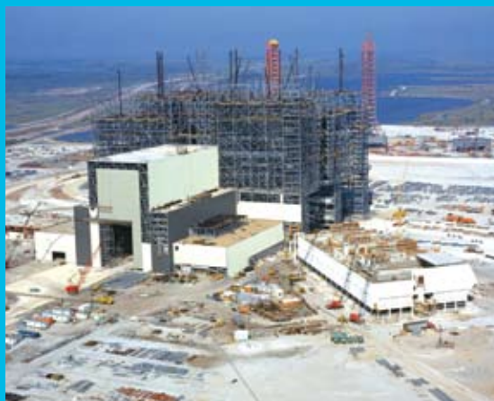
The steel framework of the Vehicle Assembly Building rises on Merritt Island during construction of America's Spaceport. The low structure at right is the Launch Control Center.
